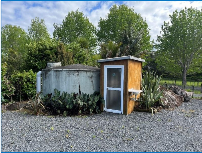
Photograph 3: Water storage tank, small building and area of wastewater treatment system.
