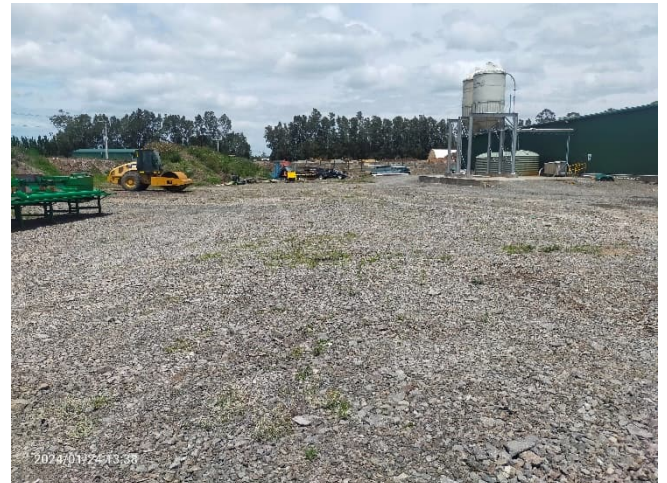
Photograph 6. View of the proposed boron plant area, looking south. Pellet plant and associated silos to right of image. Stockpile of soil with bund beyond to the left of image.
