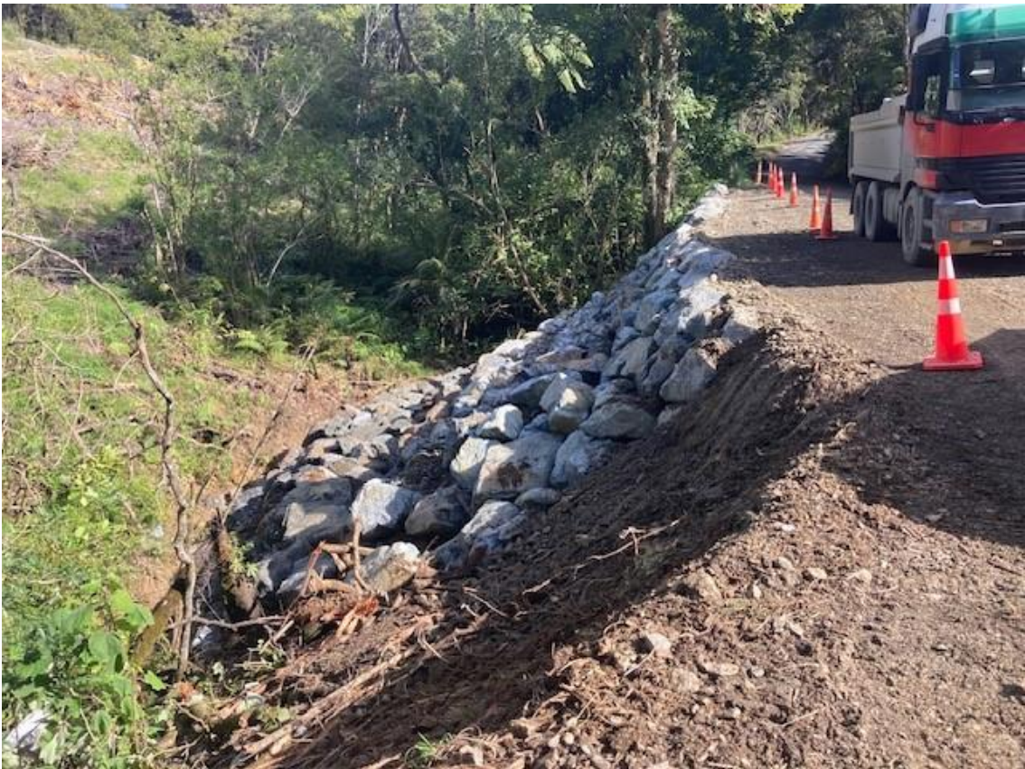
Slip repair completed on Diggers Valley Road by Mike Harrison's Digger Solutions and crew.
