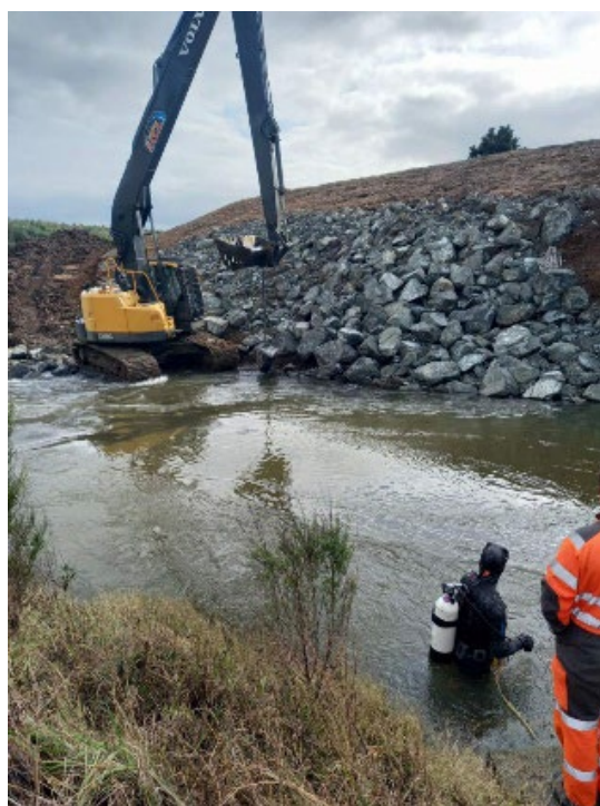
Kaitaia WTP: Awanui river intake blocking due to silt, rocks and debris, unable to supply water to the WTP.
