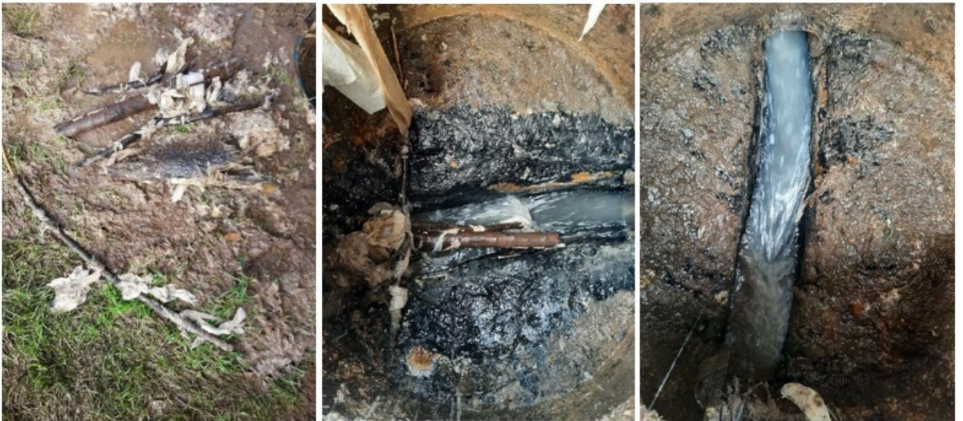
Branches jammed in at Hone Heke Rd and cleaned manhole flowing
