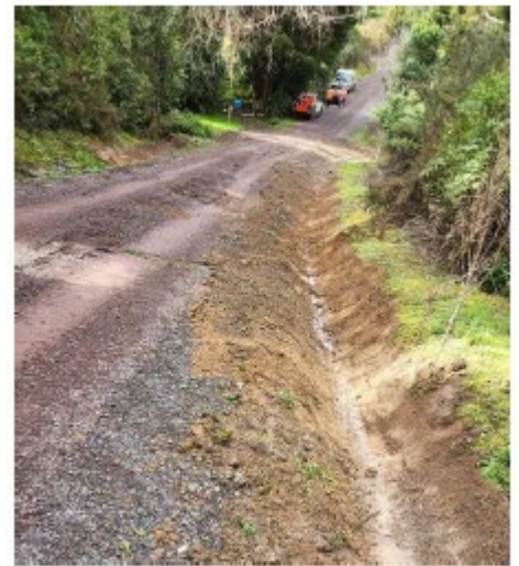
Hupara Rd – Water tabling
