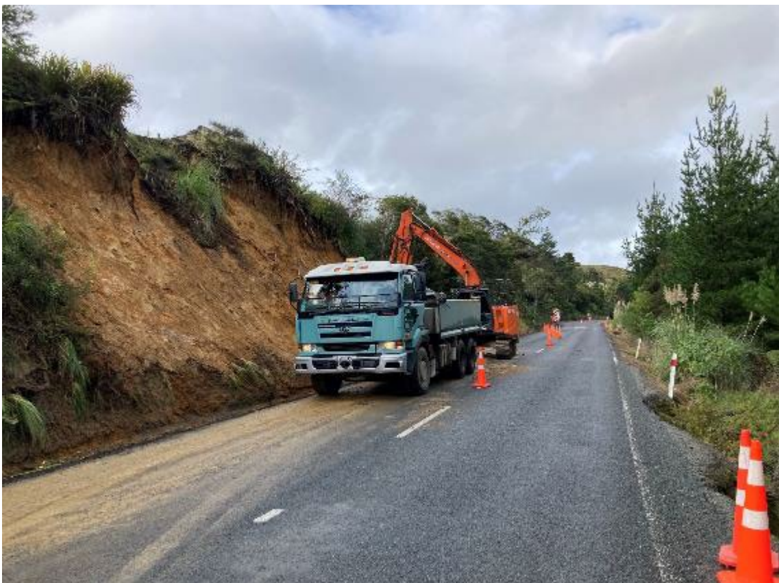
Figure 13: Awaroa Rd Slip Removal
