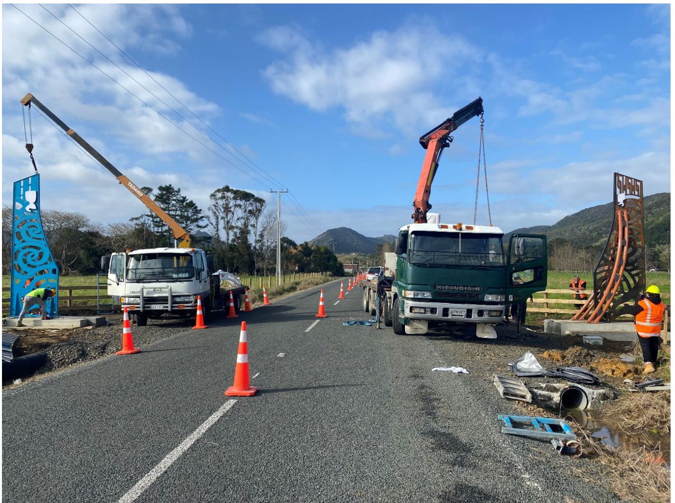
Above: Both trucks working with steel tomokanga while the stonework is being installed by Yates Transport
