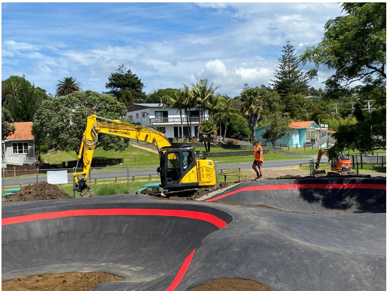
A 19 year old female digger driver from FNR did the landscaping work after the Kaitaia pump track was completed before the planting and ready lawn went down.
