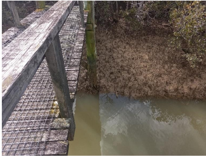
Rotten bridge pile on boardwalk section of Paihia-Opua Walkway
