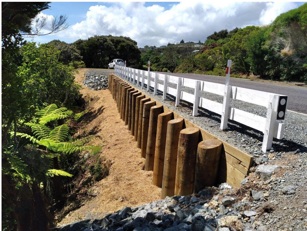
Timber retaining wall constructed at Powell Rd RP209 to prevent further undermining the road and maintain access for residents
