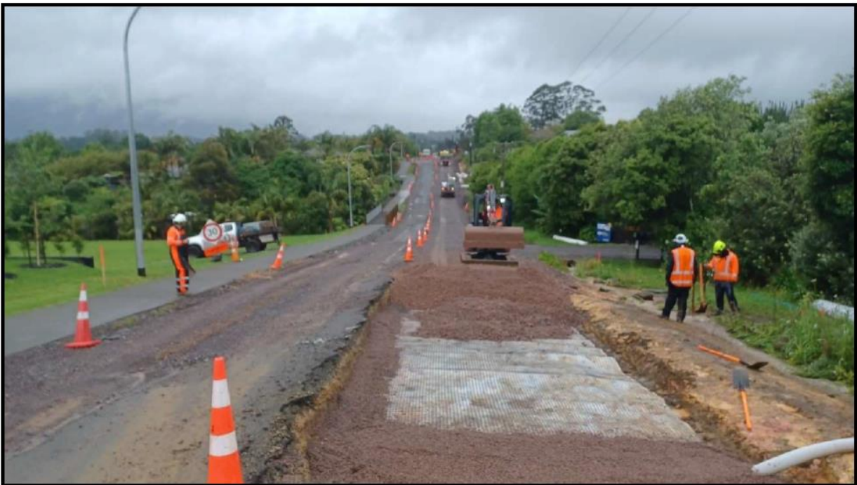
Hall Road Dig out in progress - installation of GridTex 30/30 Geocomposite, subsoil drainage and GAP65 subbase metal.
