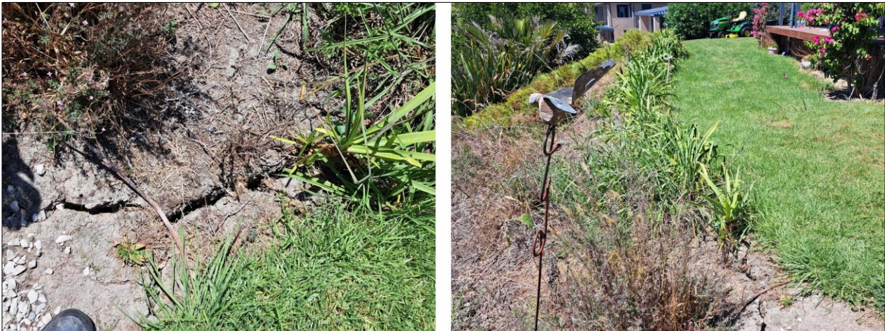
Figure 5: Site Photos – Existing Retaining Wall with obvious Cracking Observed On-Site.
