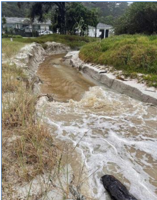
Figure 8: Stormwater flows causing scouring of beach access (Source: HG report)
