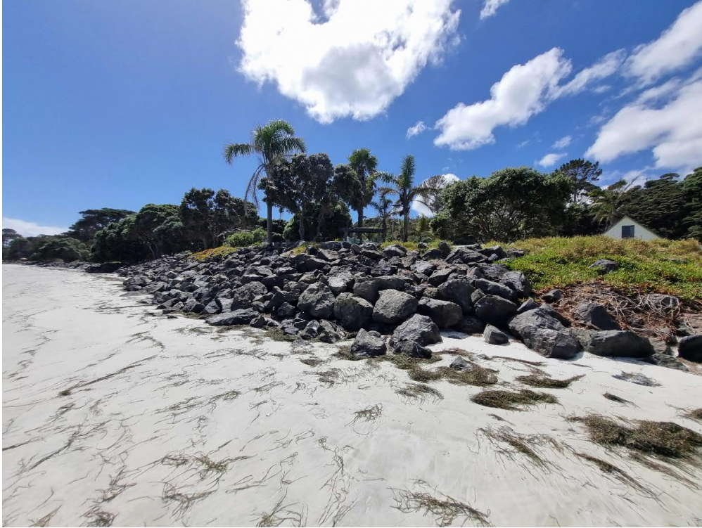
Figure B – Existing rock revetment seawall viewed from the existing southern extent of the wall at the SW corner of the property
