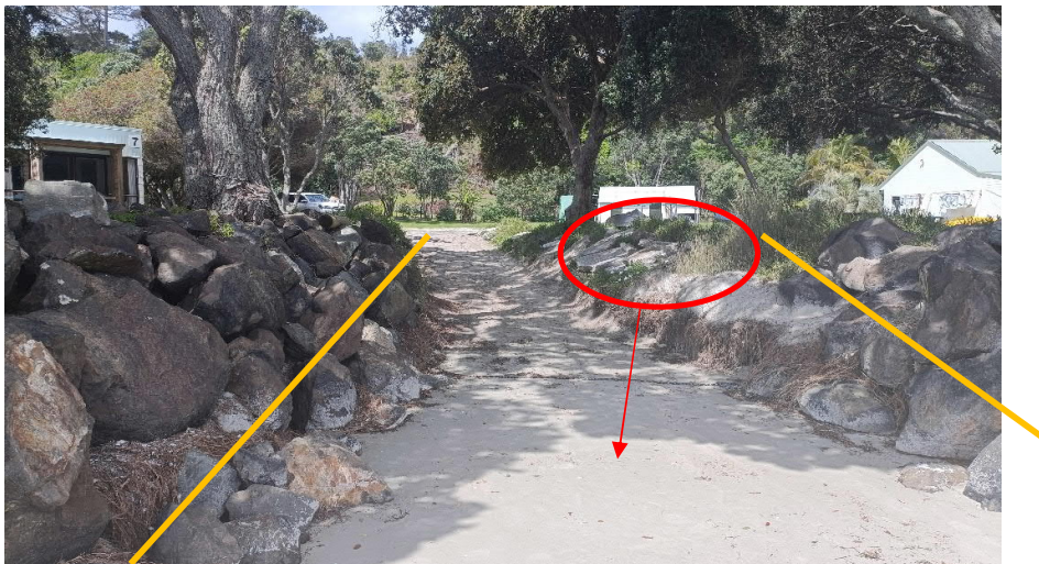
Figure L – Broken concrete (circled) will be placed in the base of the backfilled access. Approximated ramp gradient indicated.
