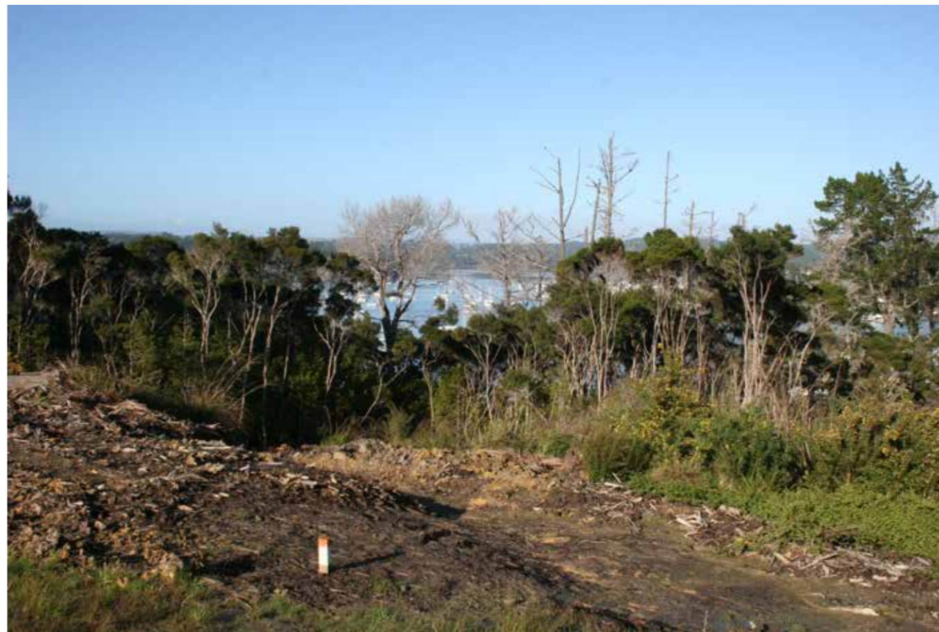
Photo 2 - View across the building site on Lot 10, and beyond to the water body around the Opuia marina
