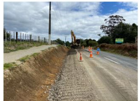
Water tabling / Shoulder Check outs – Okaihau Rd
