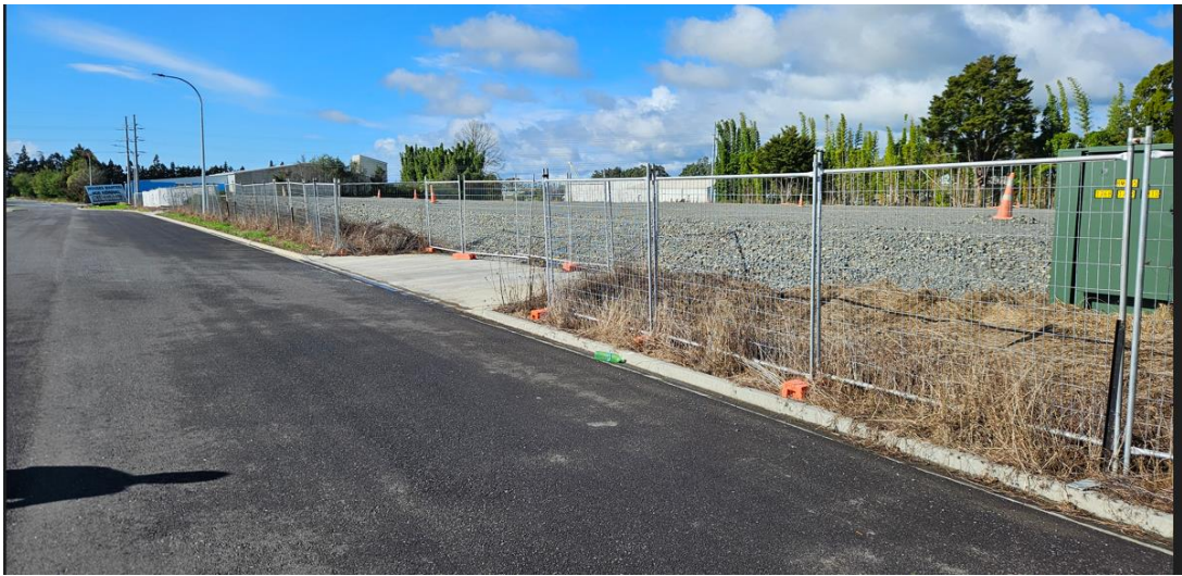
Below: The grassed eastern portion of the site in the foreground and metal building platform to the west. Beyond is the concrete batching plant and area proposed to be rezoned 'heavy industry' in the Proposed District Plan.
