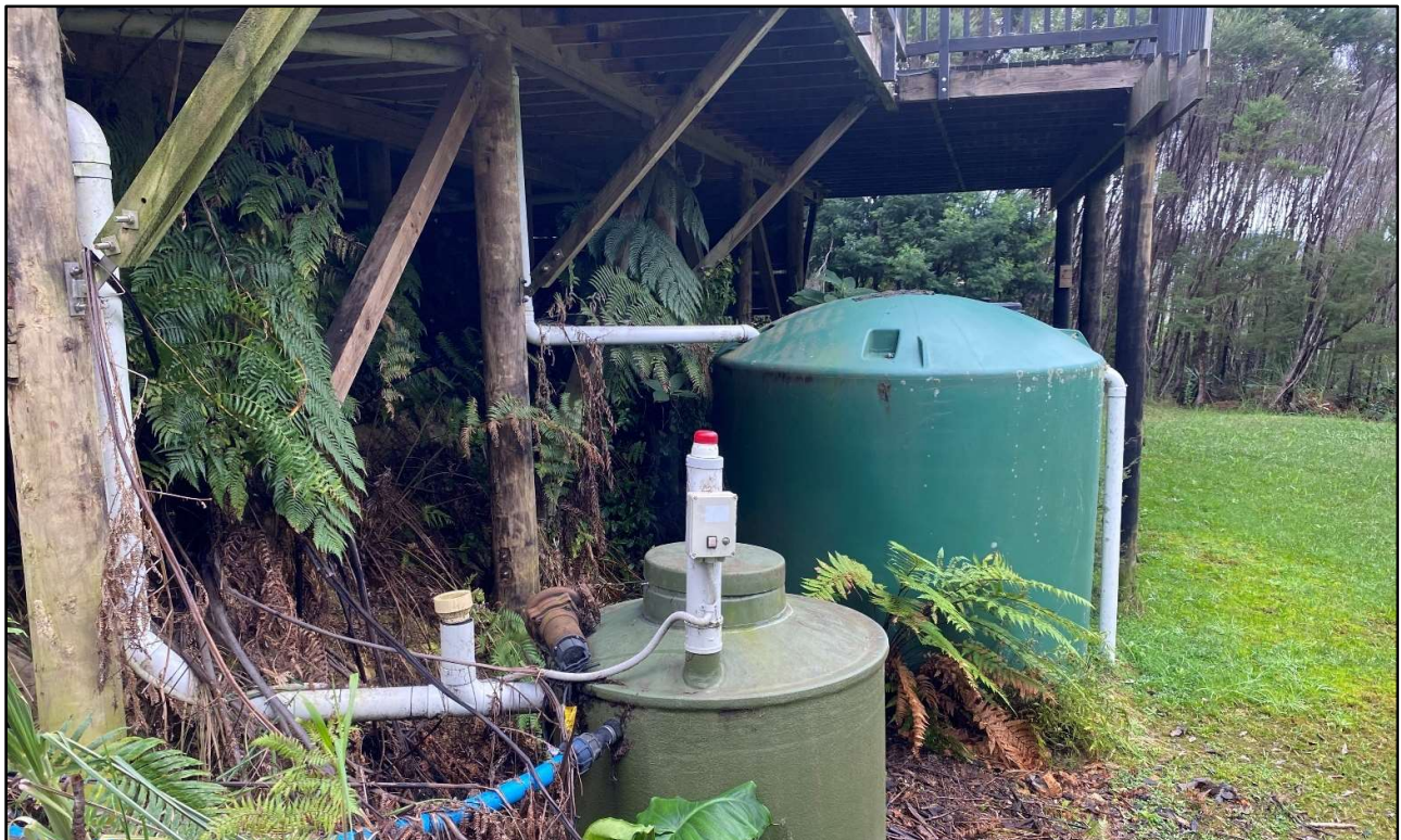
Photo – Existing attenuation tank on proposed Lot 2. Consent in 2010. 10,000 litre tank with 32mm dia Outlet pipe at base with 100mm overflow pipe at top.
