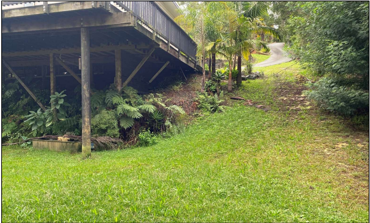
Photo – Taken from the bottom of the section looking up at towards the Northern boundary.
