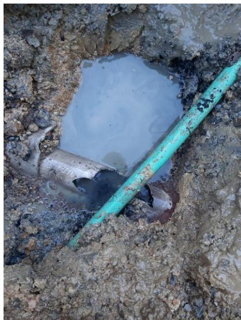
Fast Broadband duct drilled through line
