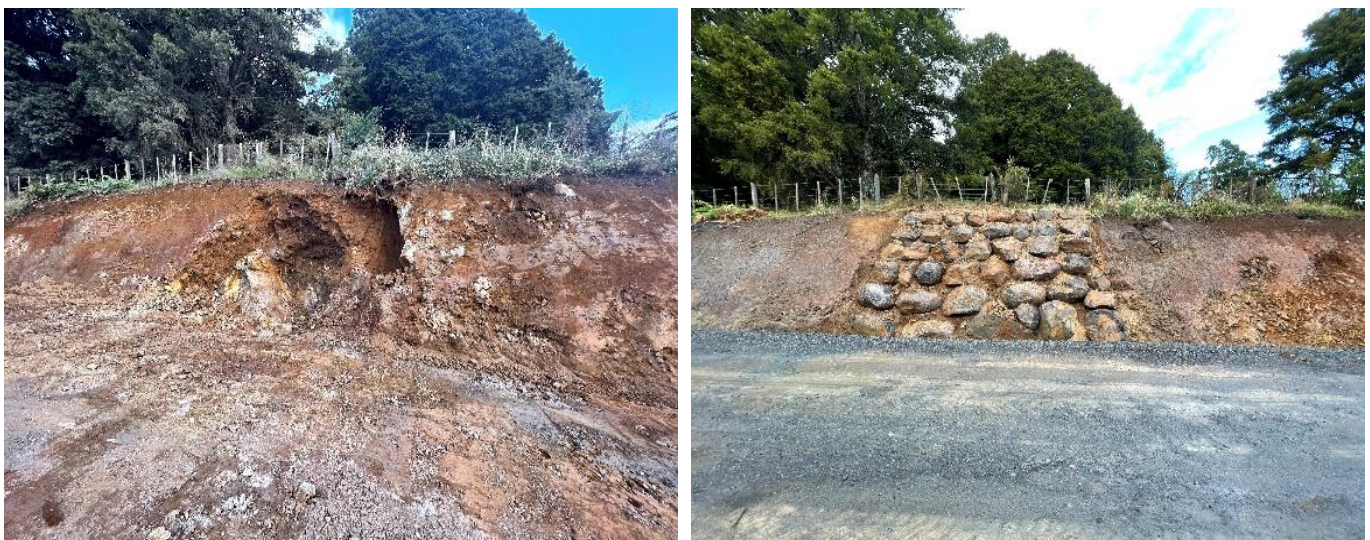
Figure 3) The photo on the left shows a large cavity after an exposed boulder needed to be relocated to allow for the road widening to be completed over this section of road. The photo on the right shows how the team have relocated smaller rocks to utilise within the cavity which provides an attractive finish as well as strengthening the existing bank surround.
