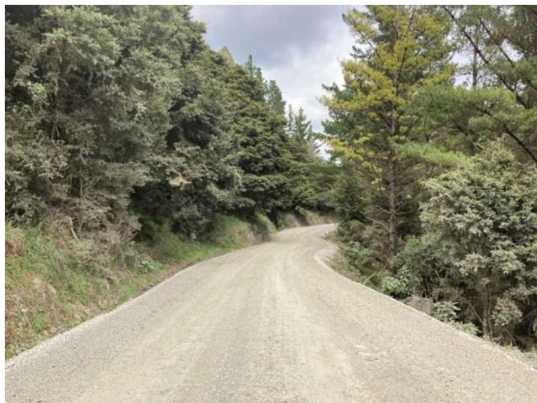
Above: Unsealed pavement rebuild on Iwitaua Road, Mangamuka. Showing super elevation crossfall through sweeping corner.
