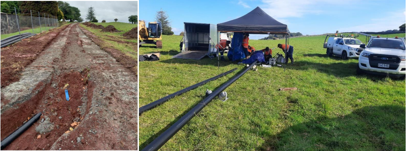
Laying pipe (left) and pipe welding (right) to the new bore – Monument Hill
