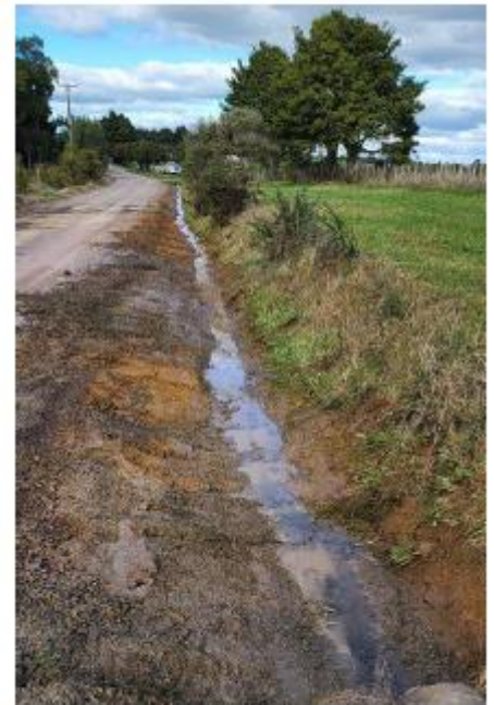
Signal Rd – Water tabling
