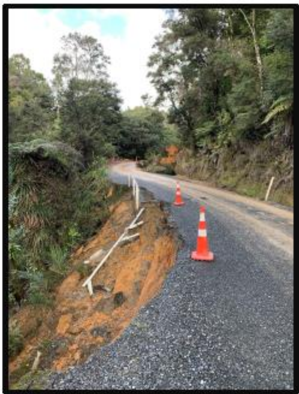
Waikare Rd – Under & Over Slip
