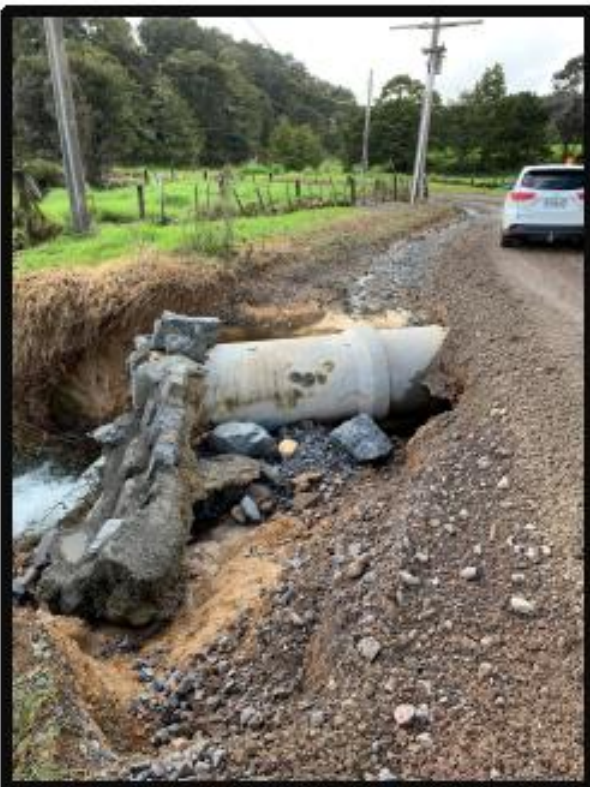
Waikare Valley Rd – 1200mm culvert wash out
