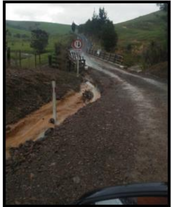
Whangae Rd – Bridge Scouring
