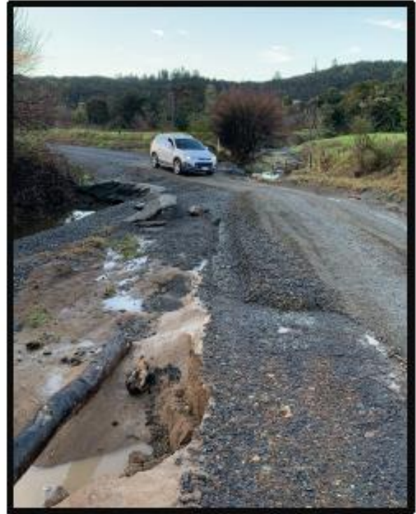
Waiomio Rd – Road Wash out
