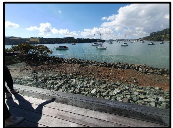
Figure 13: Image of existing natural hazard protection structures, taken from the existing deck.
