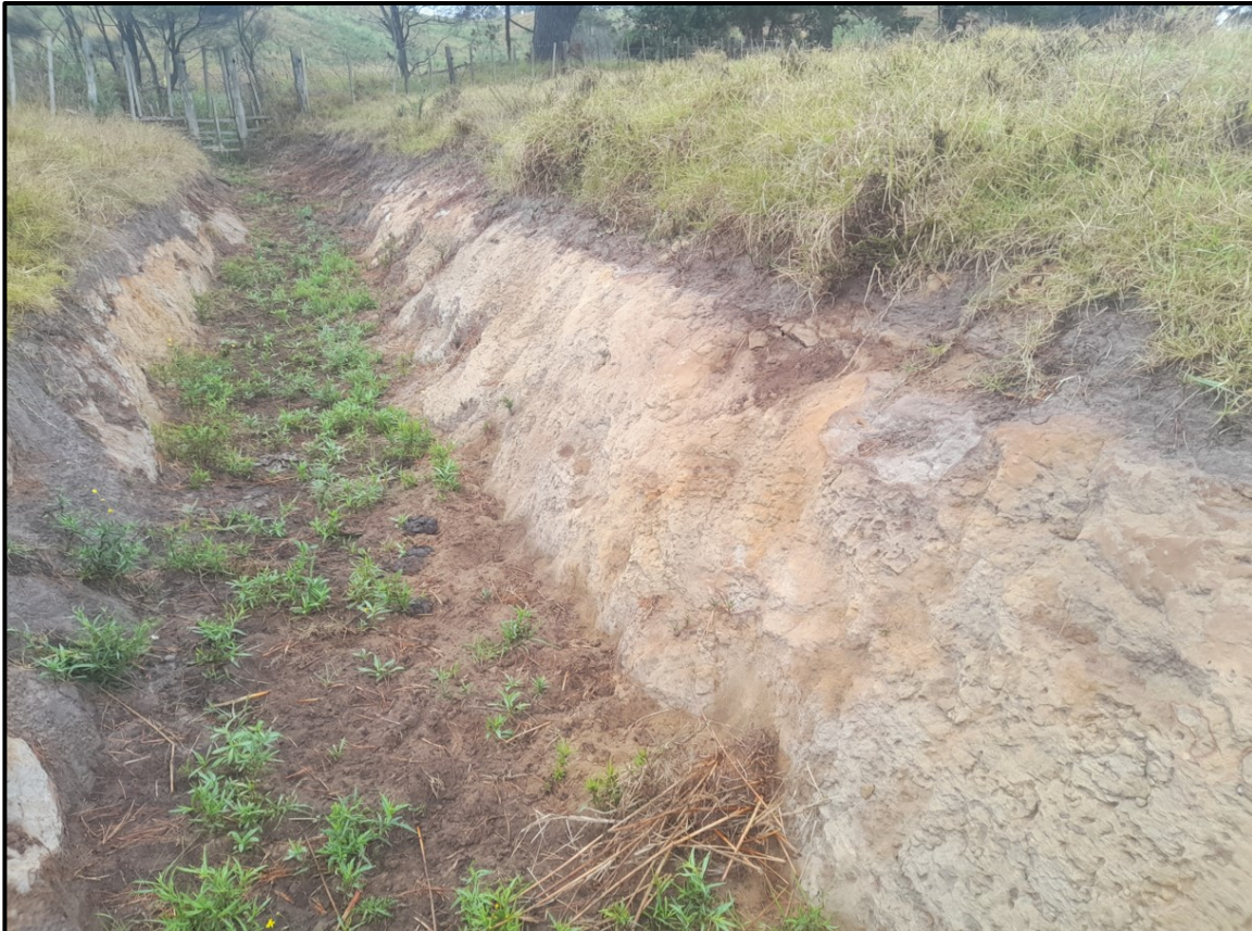
Figure 4: Exposed Sandstone/Heavily-Cemented Sand (Source: S&RC Site Photo – 13 March 2024)
