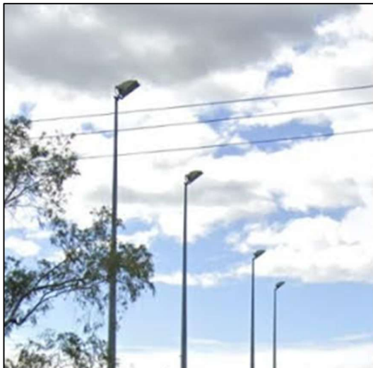
Figure 3: Lighting installed as at September 2022 [Source: Google Streetview].
