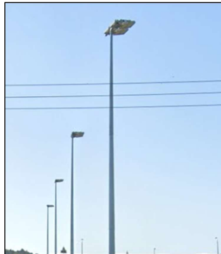
Figure 4: Lighting installed as at September 2024 [Source: Google Streetview].
