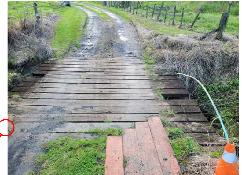
OLD TIMBER BRIDGE - TO BE REPLACED
