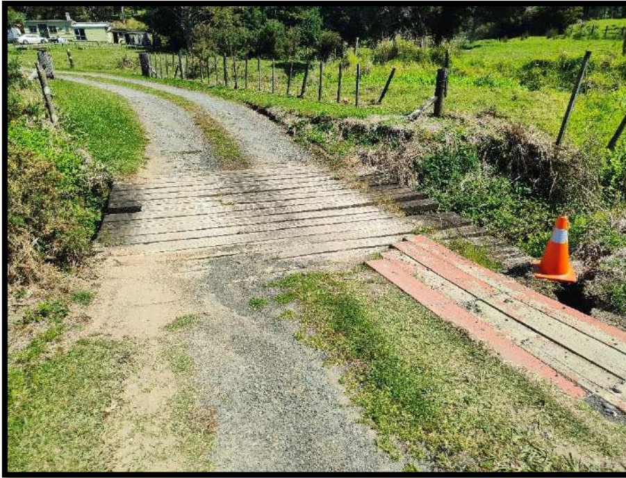
Figure 5 – Existing timber bridge within legal road, (now failed)
