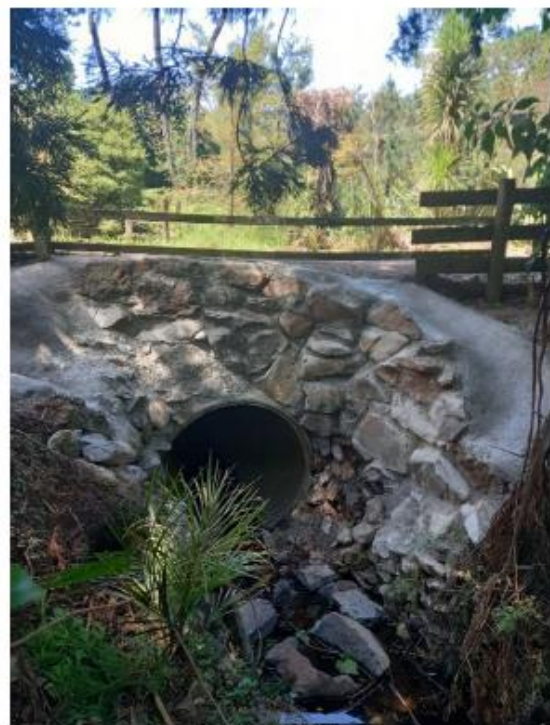
Large Headwall – Koranae Rd
