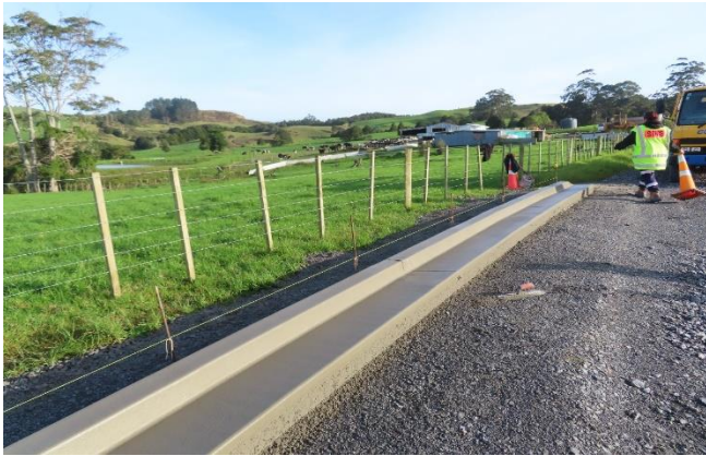
Making the most of the fine weather with the start of new kerb & channel being poured.
