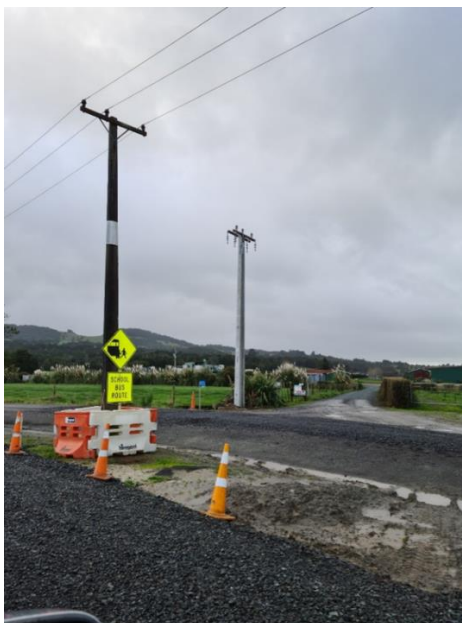
Power pole relocation at a Landowners main accessway – the old pole (left pole) is to be removed.
