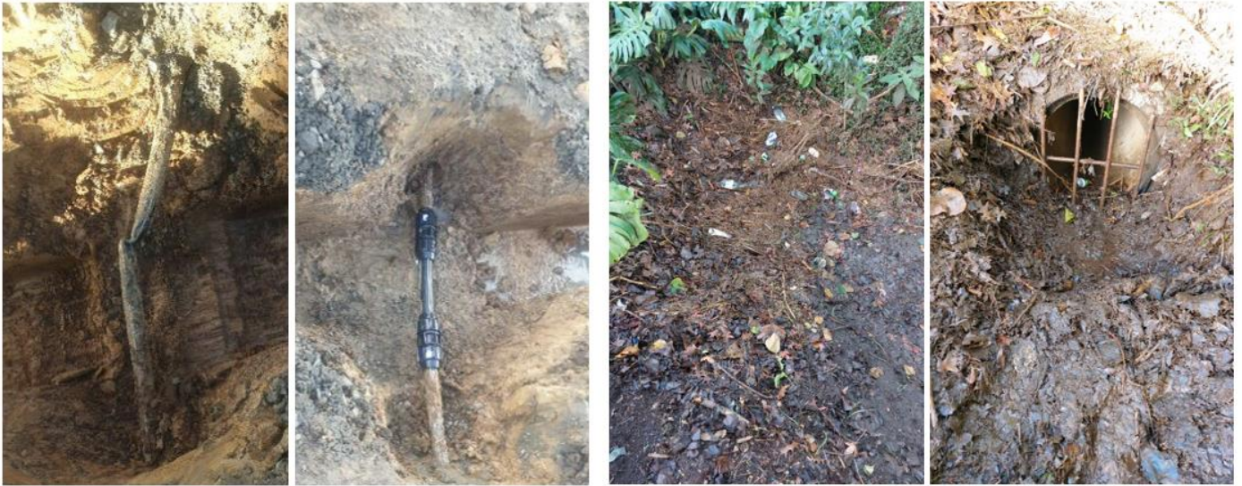
Third party damage to LPS Line.
