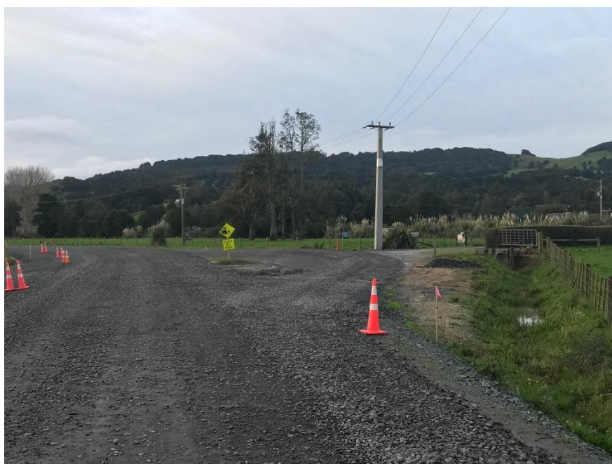
At the same location - removal of the old pole from the road carriageway with new pole installed.
