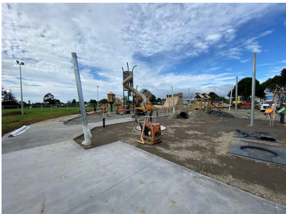
Surface levels and drainage have been set to levels to accommodate the varying safety surfacing
