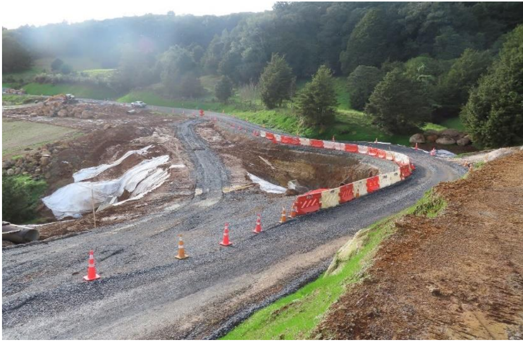
New road alignment and temporary road above the 2100mm culvert. Temporary rock stockpile to the right of the road by the trees.
