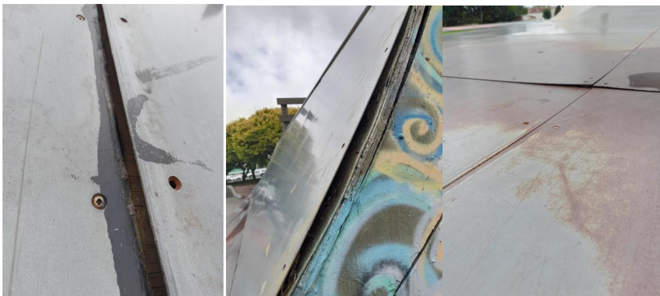
Steel plates have lifted at Skate ramp
