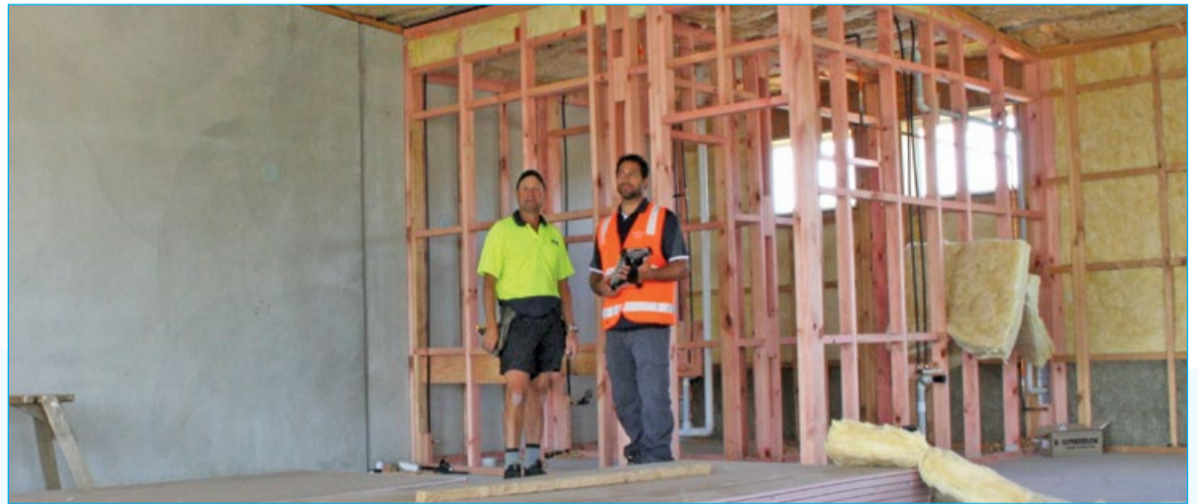
Far North councillors say new 'H1' home insulation standards are needlessly increasing the cost of building a home in Northland.
