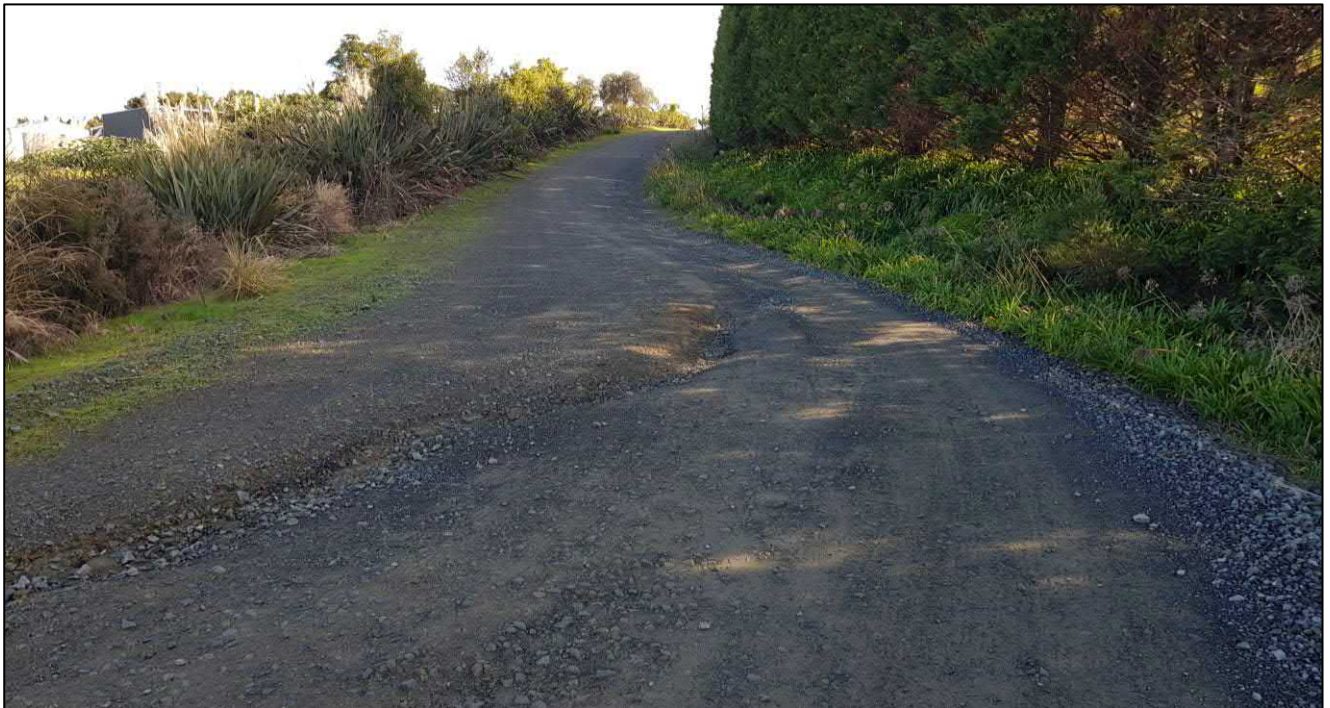
Figure 3: Arkles Way scour damage
