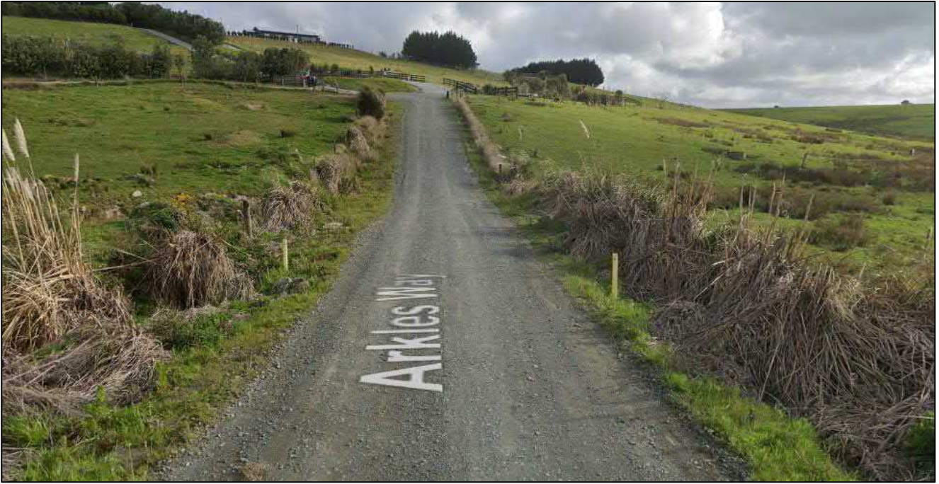
Figure 6: access showing culvert markers and carriageway in better condition (Google Street View September 2019)
