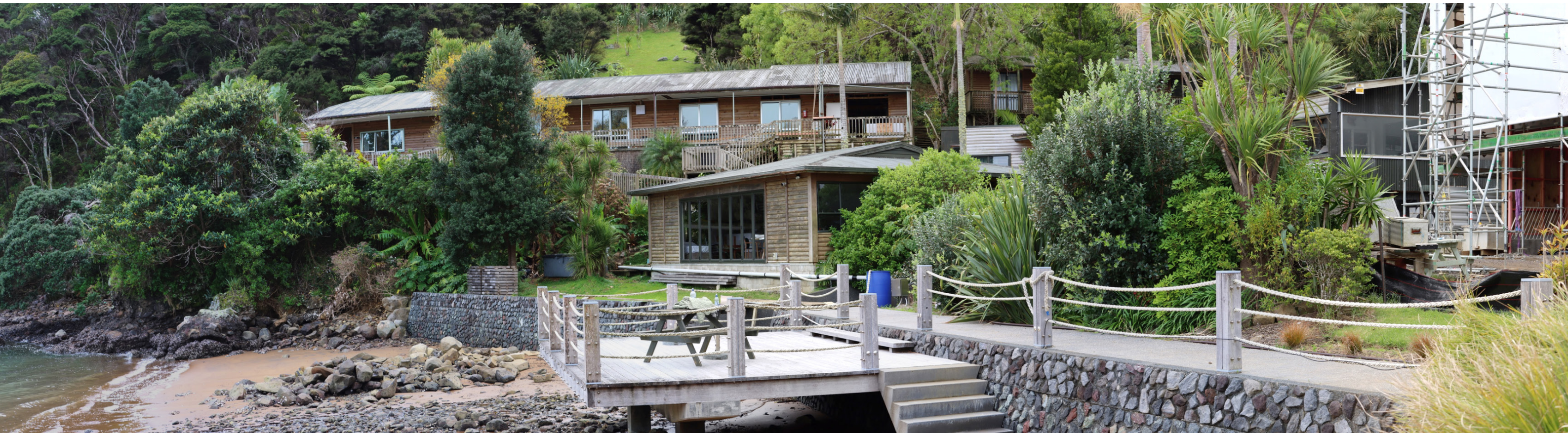
Photo 3 - View from the start of the jetty looking at the accomodation wing, conference room, deck, bar and restaurant area and the new Lodge under construction.
