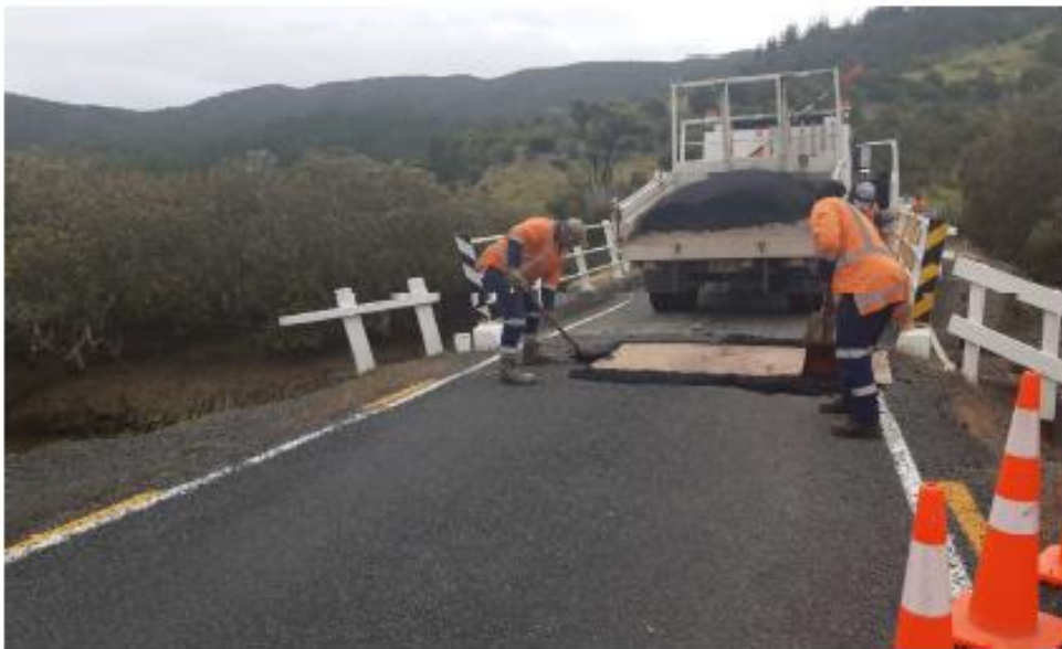
Waipiro Bay Bridge – Emergency Repairs. Final repair involves excavating to 1m down to stop abutment scouring
