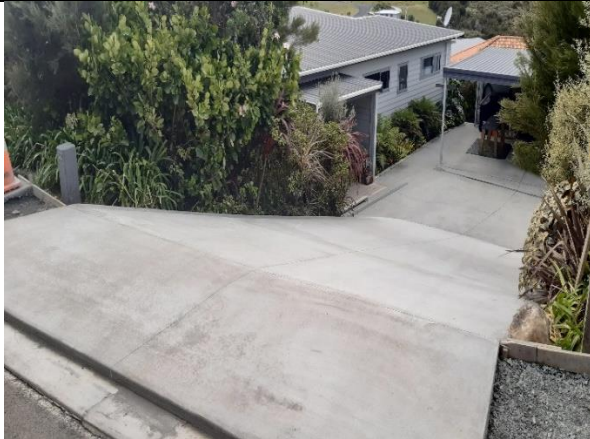
Cable Bay Block Road - Driveway reconstruction with the installation of the new footpath along
