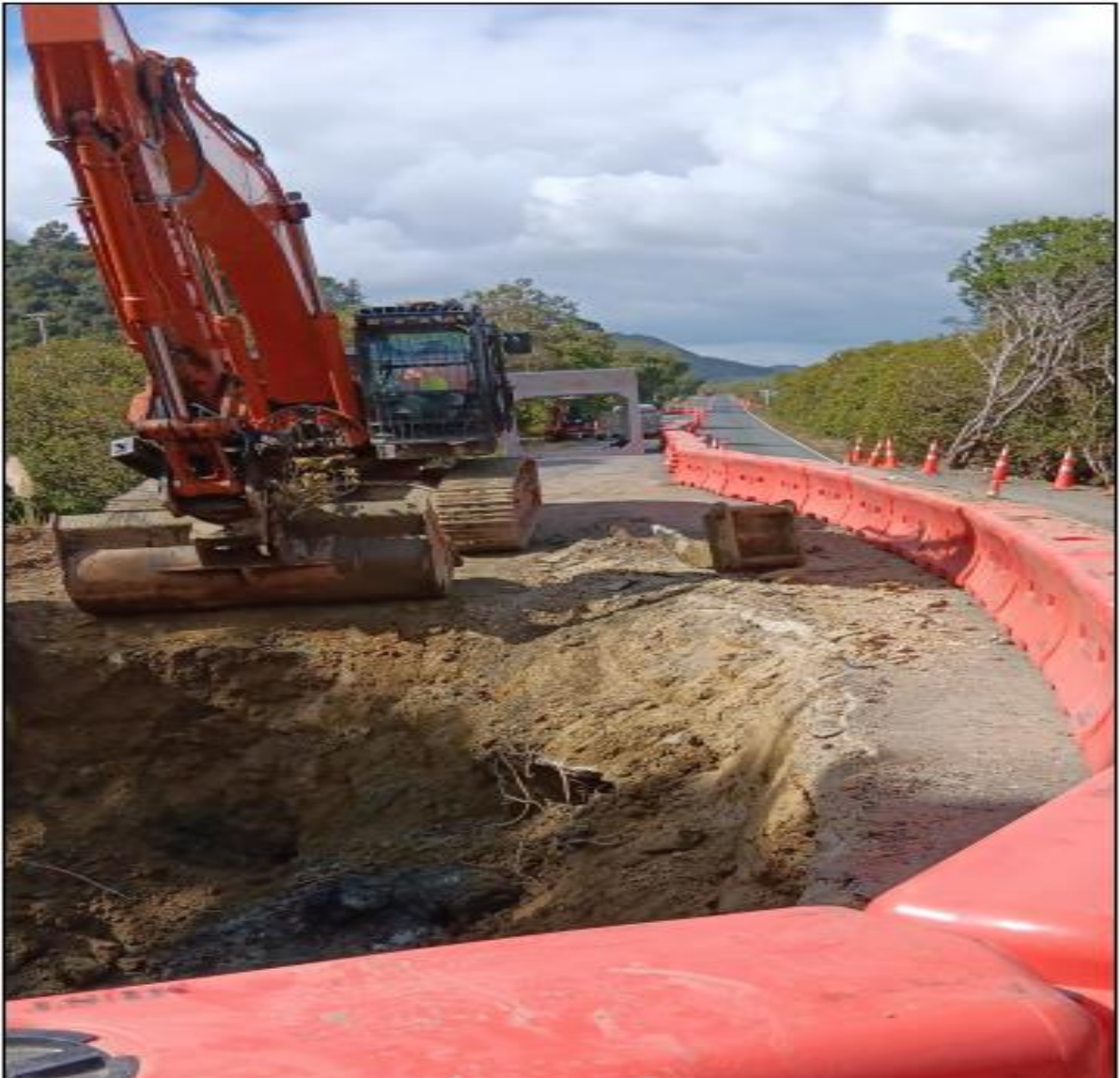
Figure 4 Whangaroa culvert replacement with portable traffic signals reducing the road down to one lane
