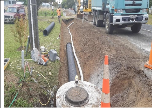
Kaitaia Awaroa Rd (Sandhills to Kaitaia) - Pipes & manholes being installed for deep swale infilling to mitigate serious safety hazard.
