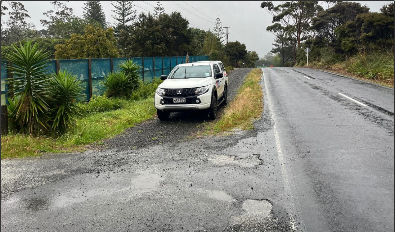
Figure 10: Site Photo 15.11.2024 – View of existing middle crossing from the northern side of the crossing, facing southwest, showing some stripping damage/wear of the crossing seal.
