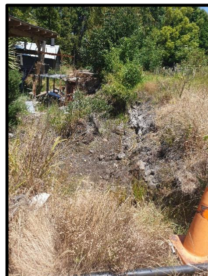
Figure 20: Drain located within Lot 5 of Stage 3 which appears to coincide with the flood area on the NRC Maps.
