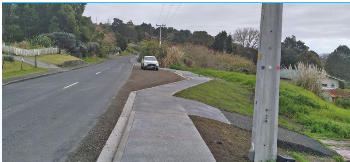
A section of the long-awaited new footpath on Parnell Street in Rāwene creates a safer route for walkers.
