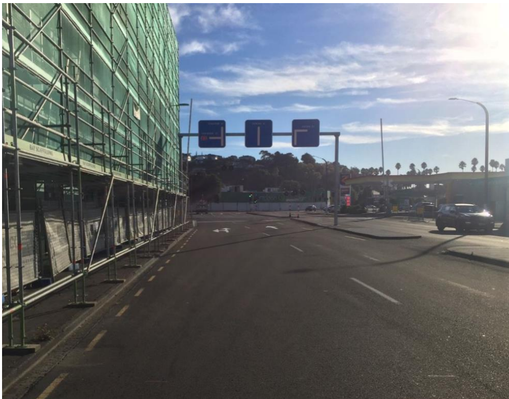
Figure 5 Scaffold obscuring signals for road traffic at a level crossing – view from the road
