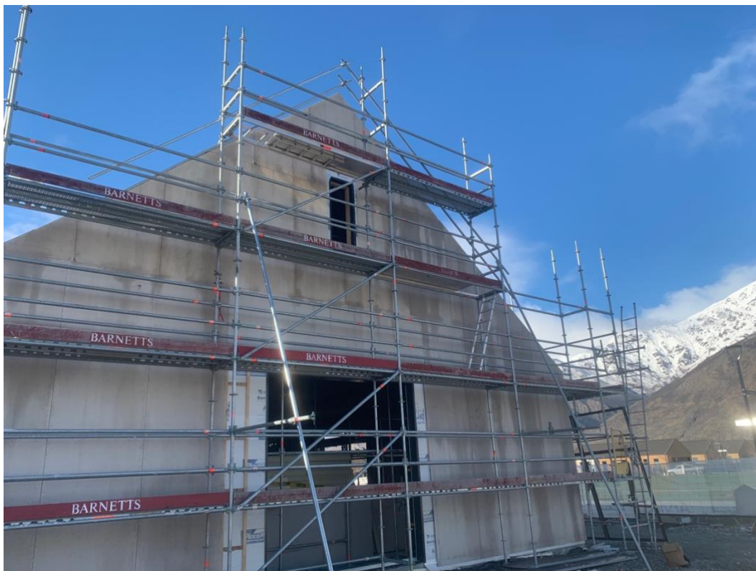
Figure 7 Photograph scaffold with outriggers, credit: Wain Chambers
