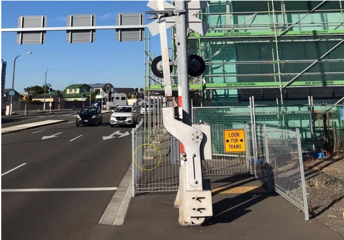
Figure 4 Scaffold obscuring signals for road traffic at a level crossing – view from rail
