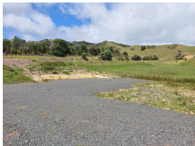
Pre-prepared building site for relocated manager's house, to the west of entrance into the site
