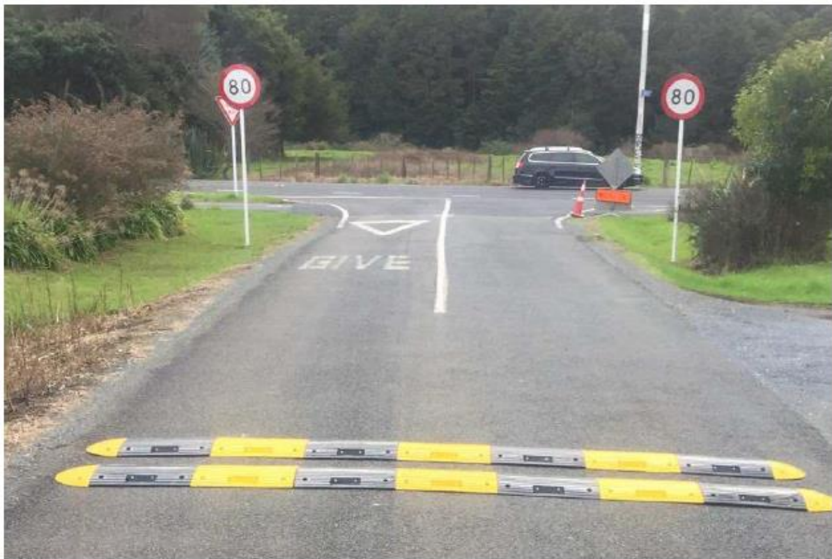
Figure 7 - Taumatamakuku - Speed Humps
