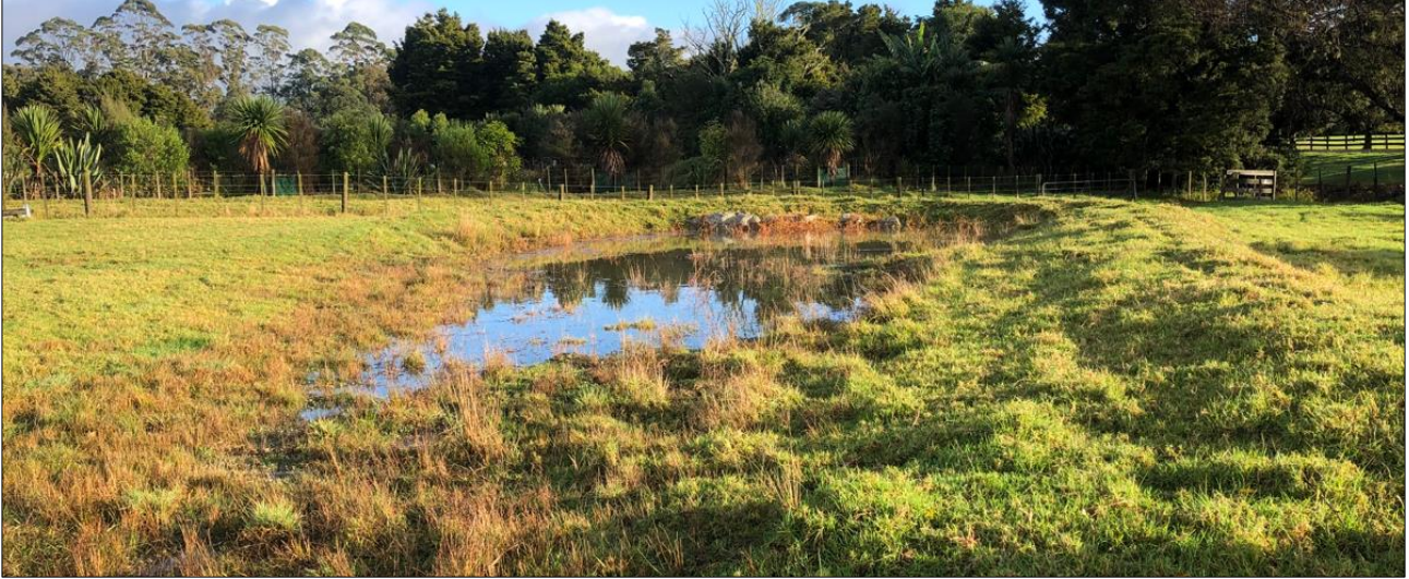
Figure 8: Site photograph of the partially filled stormwater pond, taken on the day of our investigation (northwest direction).
