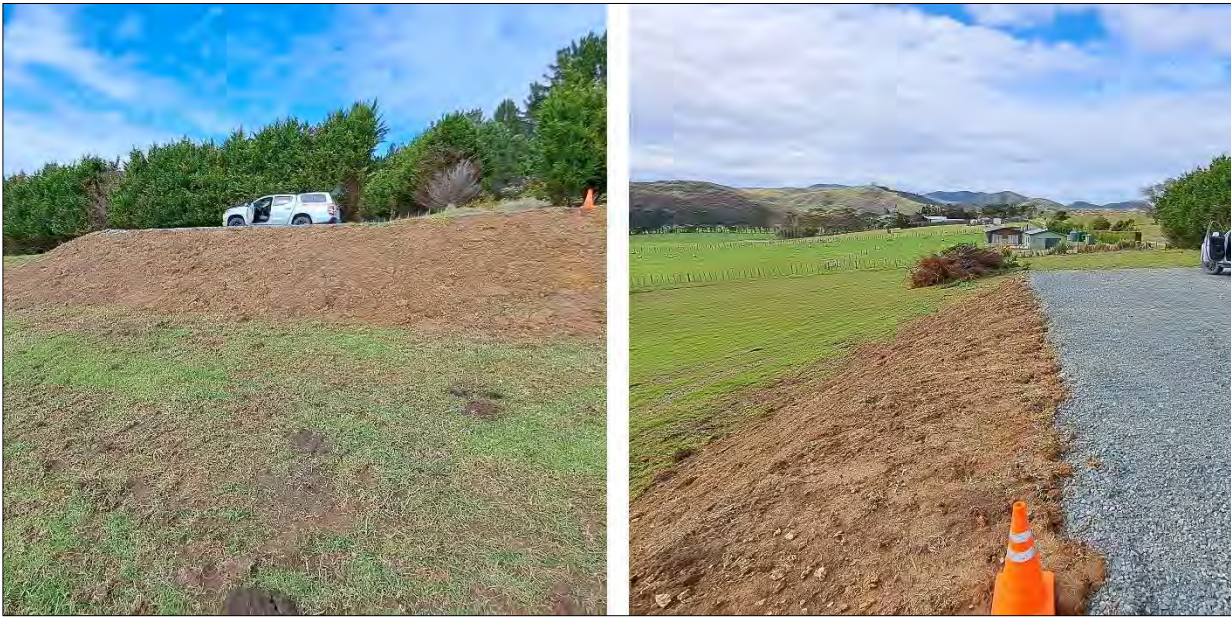
Figure 4: Site photograph of northern leading-edge of formed platform. Orange cones are indicative of proposed building site.
