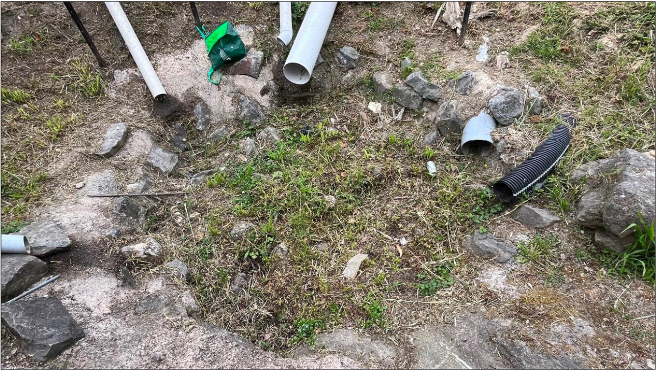
Figure 4: Site photograph of the existing inlet structure just beyond the upslope southern boundary.
