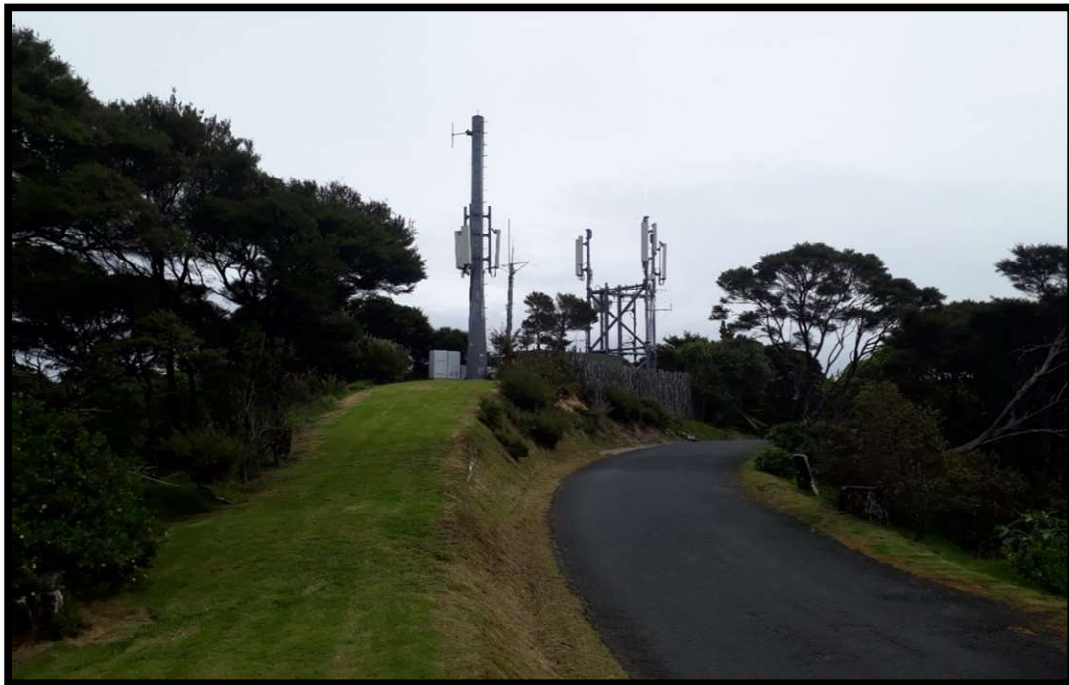
Photograph 6: Telecommunication tower on Pukematu Lane
