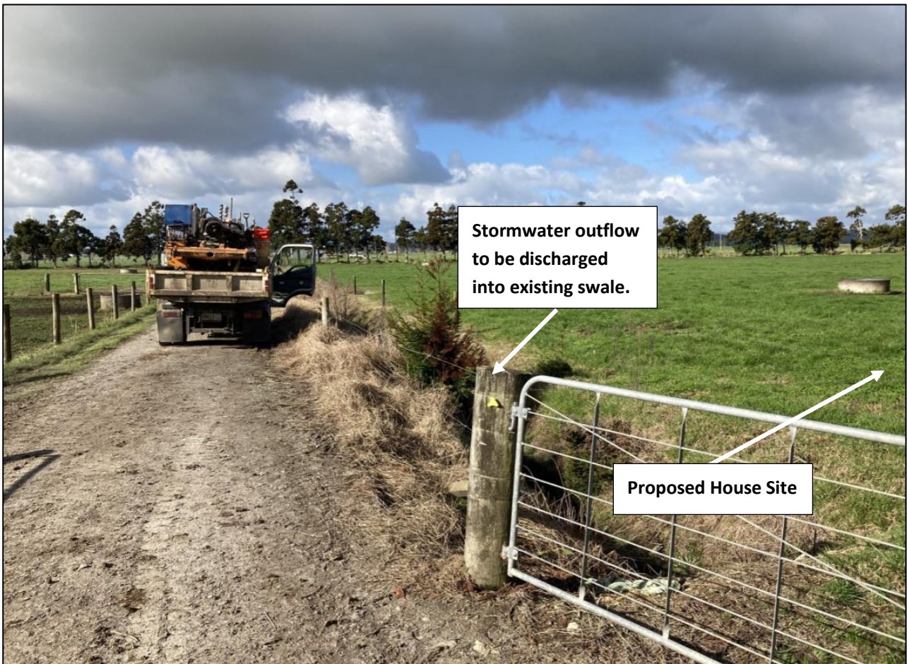
Figure 6: Stormwater to be discharged into the existing swale at 80% predevelopment flowrate for 50% and 20% AEP flood events.
