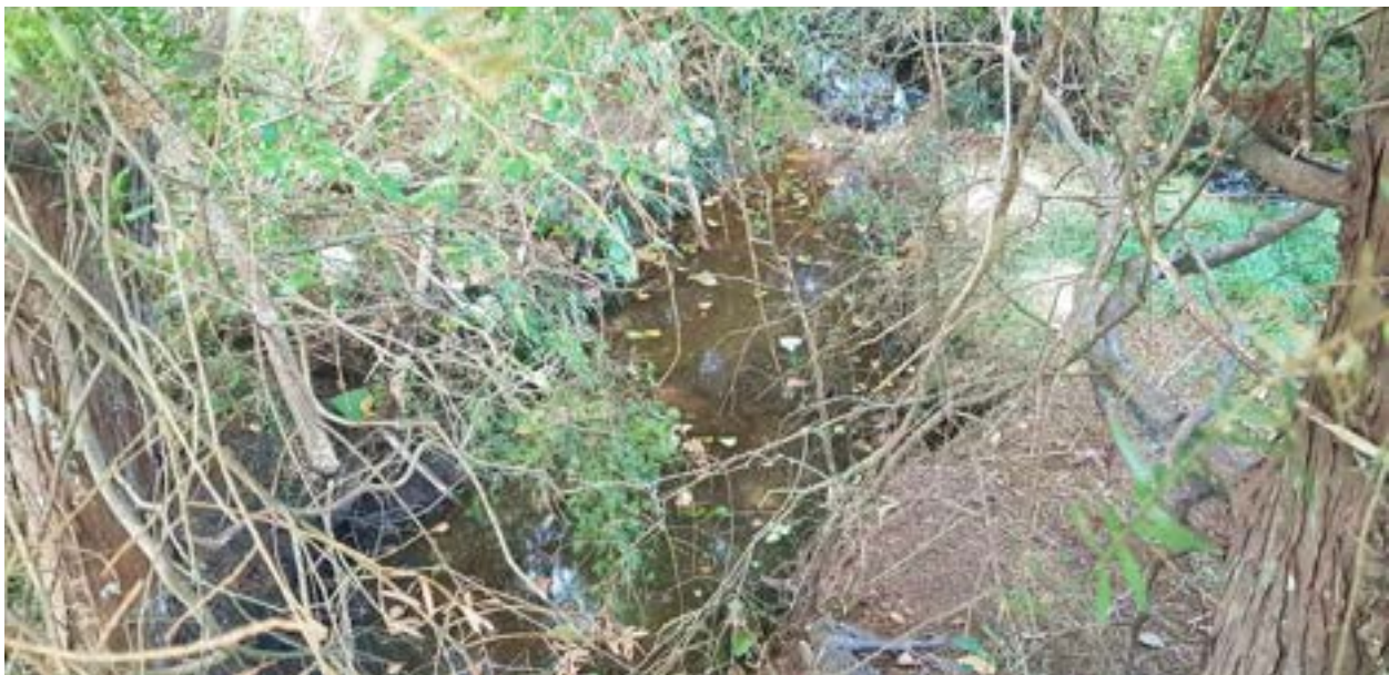
Figure 5. Stream habitat downstream of access road culvert outlet.
