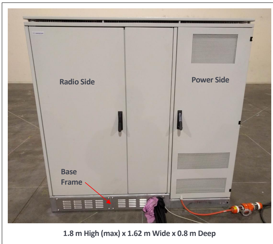
Figure 1: WCUFlex16 v2 Cabinet
