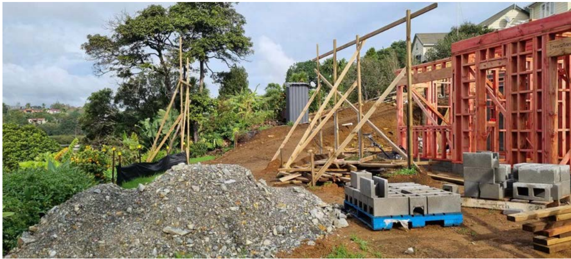
Figure 6: View looking south at reserve areas extending south in front of neighbouring properties
