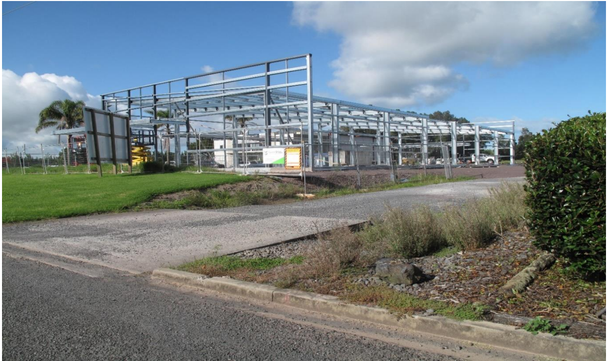
Above photo of New Commercial building under construction depicting raised building platform in Klinac Lane. Photo's taken February 2023
