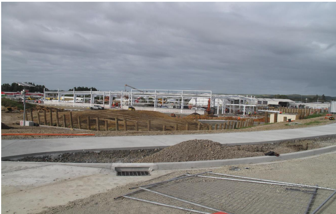
Bunnings Building under construction with the ITM Building complex in the background. Both properties feature extensive impervious surfaces that increase the stormwater flows to the Waipapa and Kerikeri river catchments.
