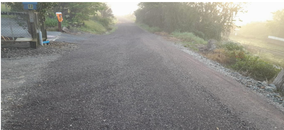
From site crossing (bottom left hand corner) looking eastwards back towards 'town'.
