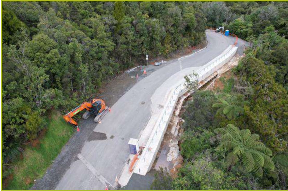
Figure 6: Example of Typical Slip Site (Slip A5 Near Completion of Remediation Works (Image Taken: 6 August 2024))
