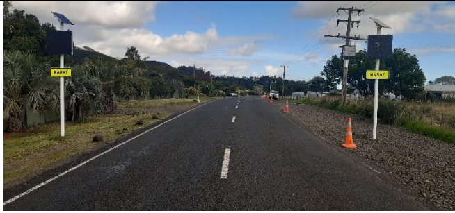
FNDC Contract 7/21/216 – HRRR Corridor Safety Treatments & HRI Intersection Safety Treatments - VMS signs installed
