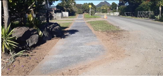
FNDC Contract 7/23/185 - FNDC Footpath Projects Suite 3 (21-24) New Footpath along Takahe Rd in Ahipara upper end
