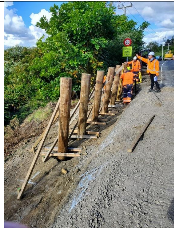
7-23-188 School to Honey Street section, Rawene. Retaining wall post for new footpath, inspection.
