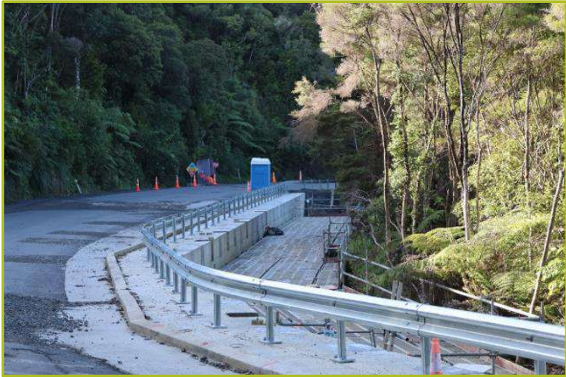
Figure 7: Example of Typical Slip Site (Slip A3 Near Completion of Remediation Works (Image Taken: 14 August 2024))
