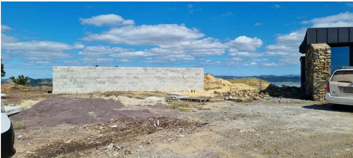
Figure 5: View of the garage building site (in front of the wall). The area behind the wall will be landscaped to screen the garage from the coastal aspect.
