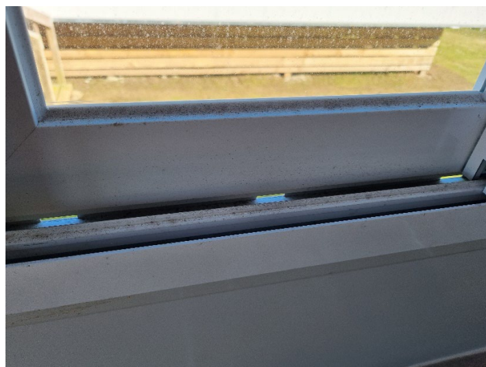
Figure 10: Condensation drains (internal)
