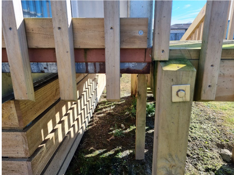
Figure 14: Corrosion to deck structure
