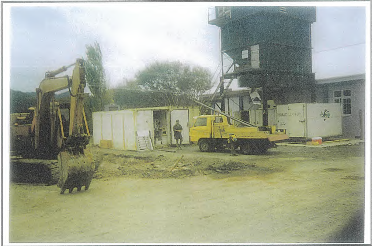
Photo 1: View of the tank-pits. Estuary to left/rear of photo, SH10 to the right.
