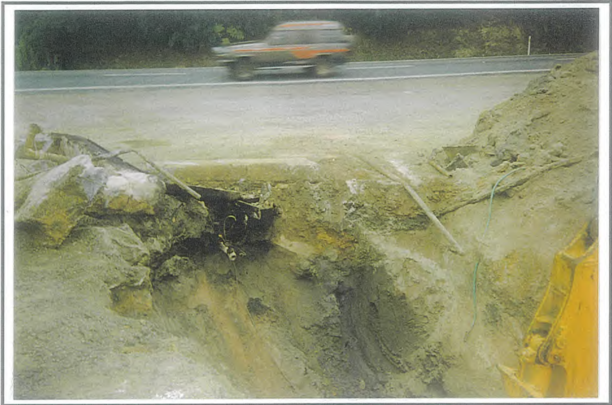
Photo 5: The tank-pit after removal of the second diesel tank. The pumps were located at the end of the pit, and the dark soils beneath them were removed.
