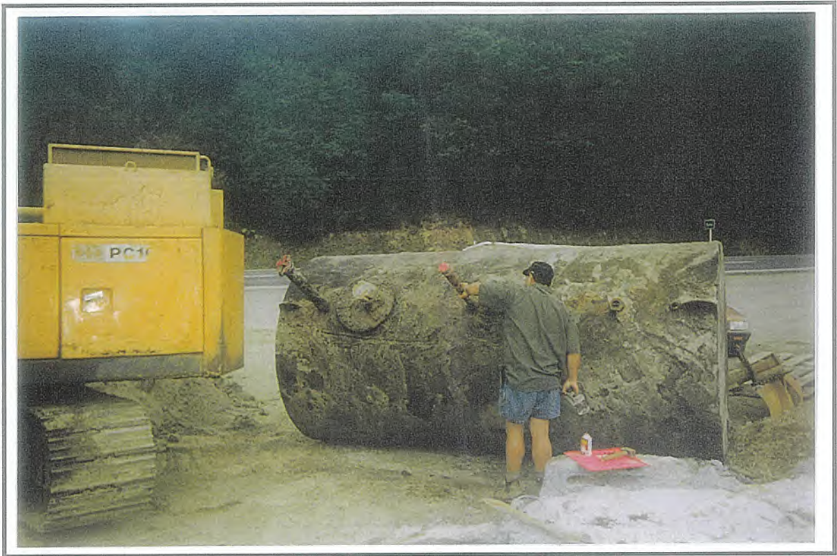
Photo 3: The second 9,000 litre diesel tank (TP2).
