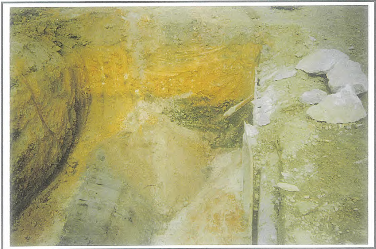
Photo 4: The tank-pit after removal of the first tank, showing the base material that was subsequently removed.
