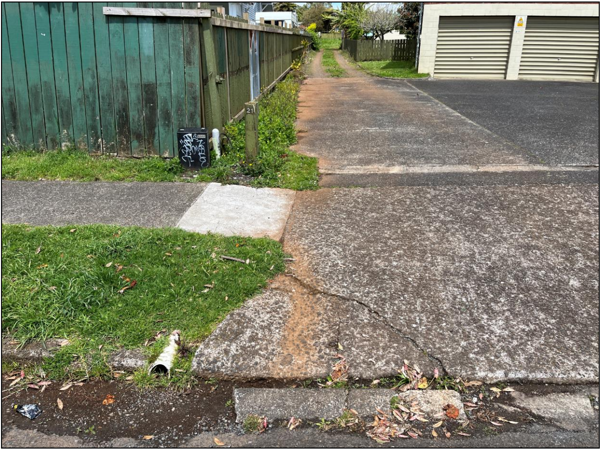
Figure 4: Driveway into the Site showing the 100mm diameter stormwater pipe to kerb
